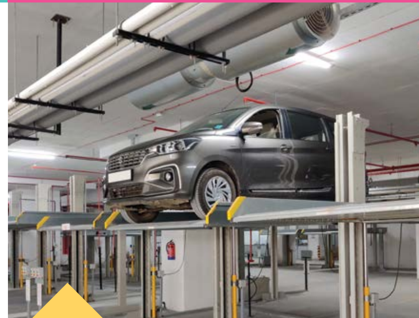
Stack parking option is provided in the basement, wherever feasible, thanks to generous slab heights.
